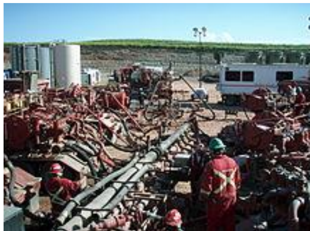
Fig. 10 View of surface equipment at a typical Fracking Well installation
